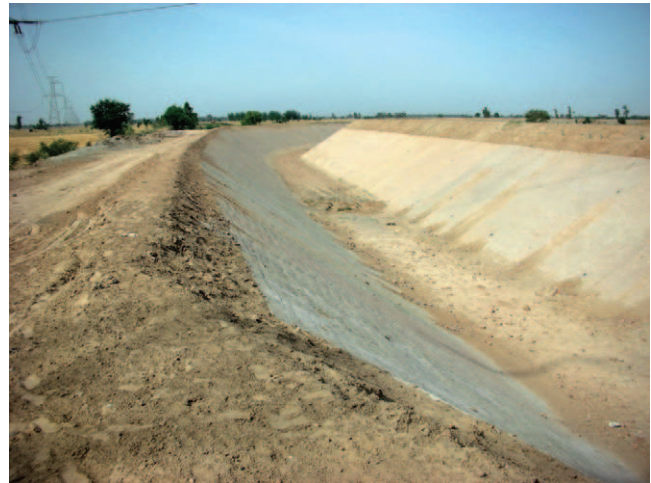
Figure 4.8 A lined irrigation canal in Haryana, India. Such lining is an important way in which to reduce waterlogging and salinization. (See Plate 26)
