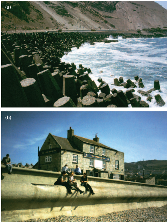
Figure 6.28 (a) Coastal protection measures at Arica, northern Chile. (See Plate 45) (b) A sea wall on Portland, Dorset, southern England. (See Plate 45)
