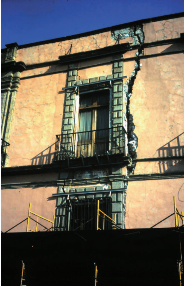
Figure 6.13 The city of Mexico has subsided by many metres as a result of groundwater abstraction. Many of the ancient buildings in the city centre have been severely damaged, and have been cracked and deformed. (See Plate 40)
