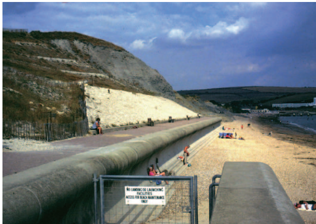
Figure 6.24 Coastal defence in Weymouth, southern England. The piecemeal emplacement of expensive sea walls and cliff protection structures is often only of short-term effectiveness and can cause accelerated erosion downdrift. (See Plate 43)
